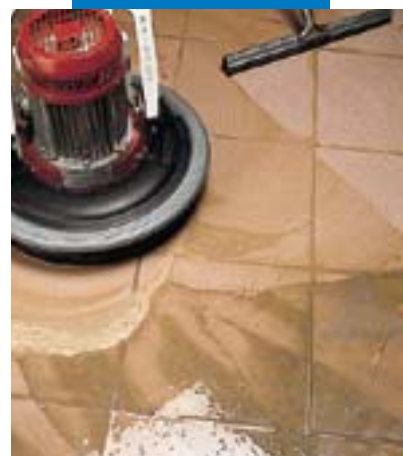
Finishing a porcelain tiled floor with single-brushed power float or rubber rake
