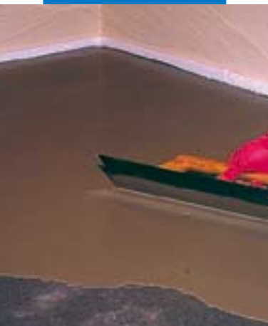
Applying Novoplan 21 with a metal trowel on a cementitious screed primed with Primer G
